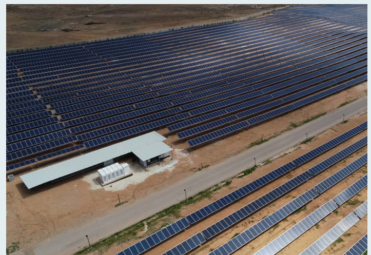
Figure 9: Al Badiya Storage Expansion project (23MWp/12.6 MWh).
