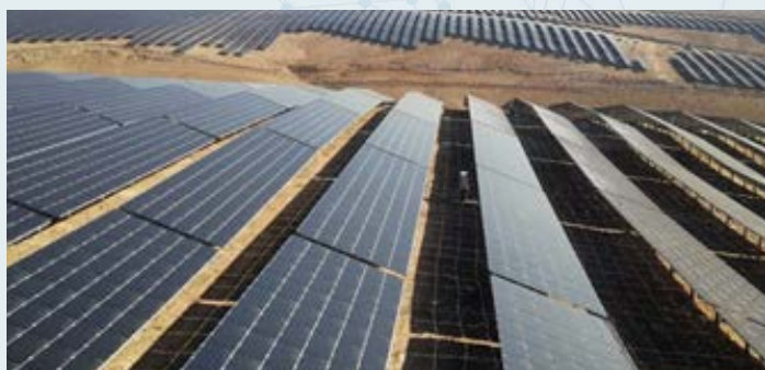
Figure 11: South Amman Solar Power Plant.
