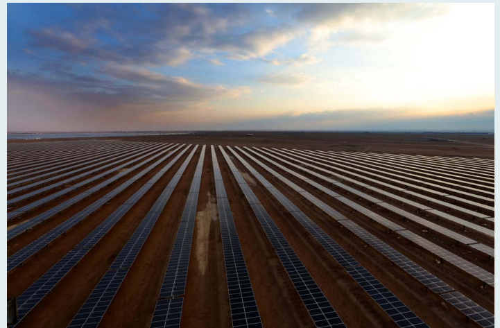
Figure 7: Solar PV Power Plant (Source Kawar Energy Company - Orange Project).
